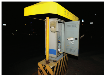
Traffic signal controller
