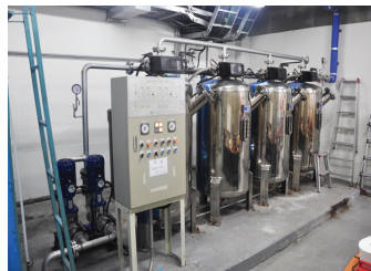
Water purification facility panel board
