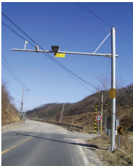
CCTV panel board
