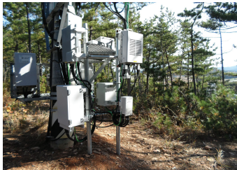
Communication repeater panel board
